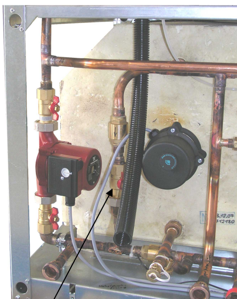
Stop-ball-cock in the dual differential pressureless manifold
